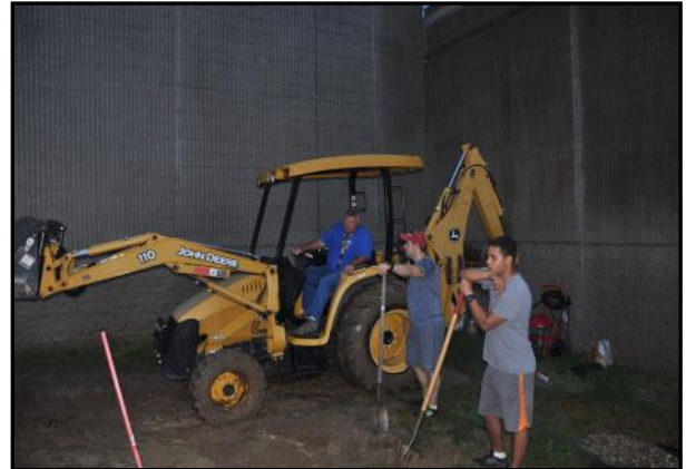
Foreman Todd Spencer ensures work is done to specification and gets in a little “machine therapy” before his heavy equipment license was revoked
